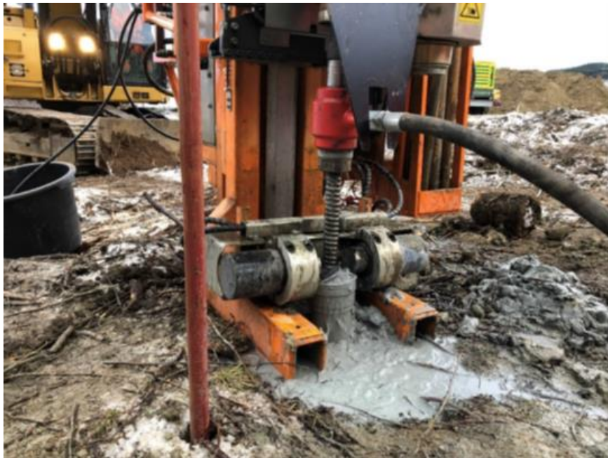
Figure 94 Installation of salt injection well for stabilization of quick clay in Tiller-Flotten
